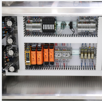
Hopper Control Panel: Current Industrial Controls
